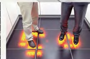
Shuttle elevator (floor lighting)
