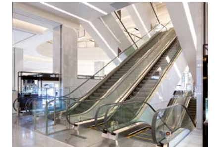
Hyundai Department Pangyo Store 82 escalators
